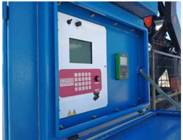
Figura 23. Pump Off Controller y VDF.
